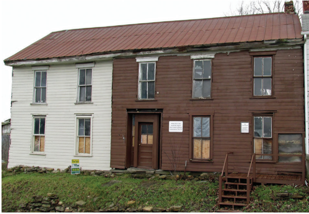
With its log walls wrapped in wood clapboard, the original Ohio County Courthouse still stands about 12 miles north of Wheeling. It was constructed in 1778 - 1779 but is severely deteriorated and for sale. Photo by Earl Nicodemus.
